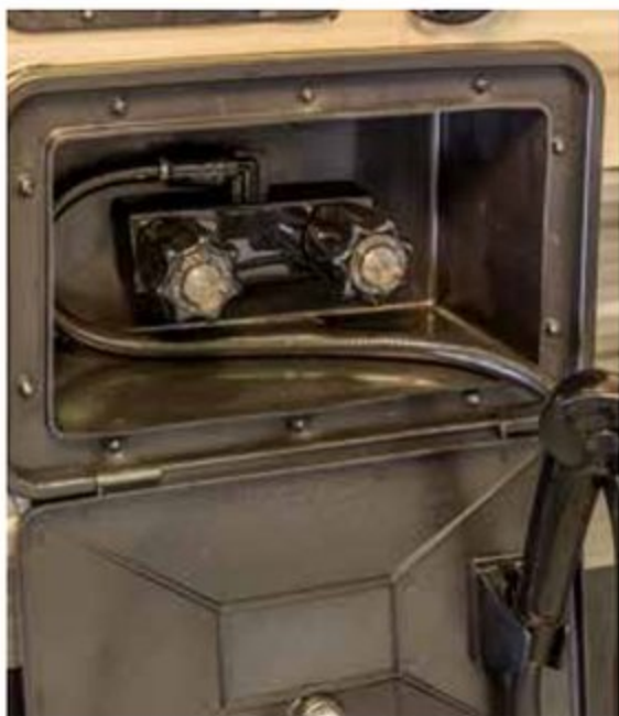
Outside Shower With Hot And Cold Water
