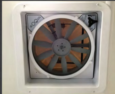
High Output Attic Fan in Bathroom
