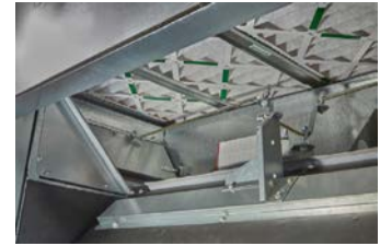
Economizer, No Controls
