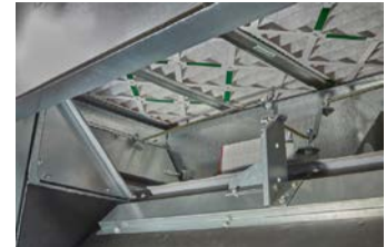
Economizer, Jade Control
